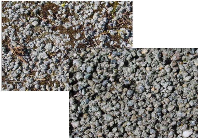
Cleaning of clogged pervious concrete (upper left) can restore 90% or more of the original permeability (lower right).
